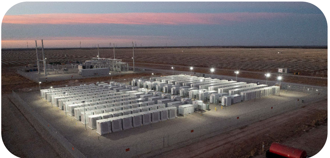
Figure 1. Example of a BESS Project
