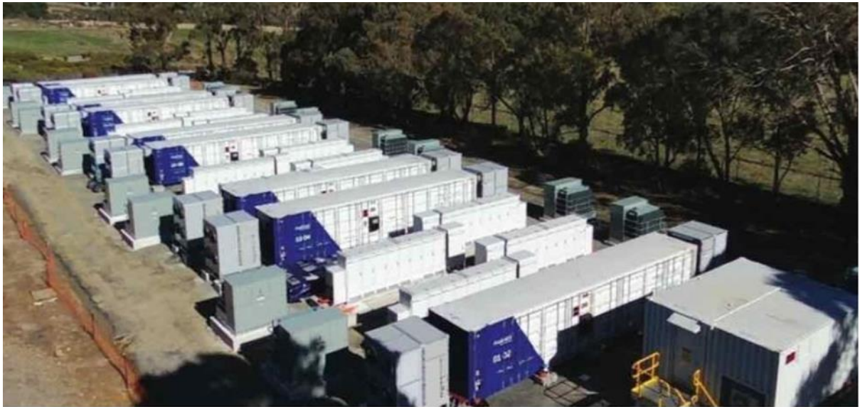
Figure 11: Containerised Battery Storage System
