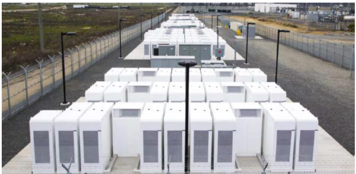
Figure 10: Tesla 40 MW Powerpack System
